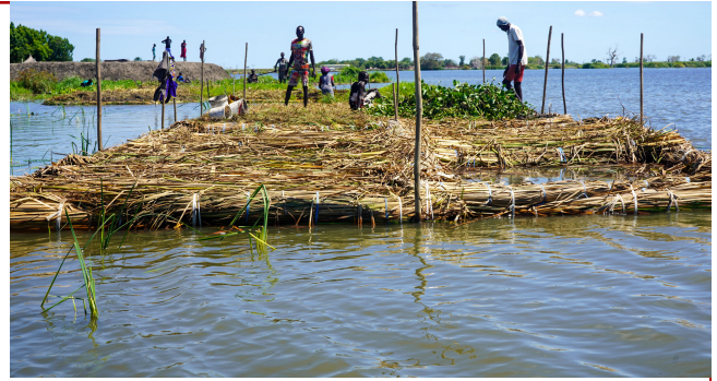
On going construction of floating gardens amidst the floodwaters of Rubkona, in South Sudan.
